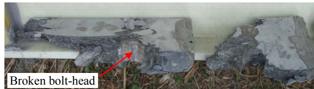
Fig. 2.13 Broken FRP bolt-heads in G10-F16-BN4 beam
