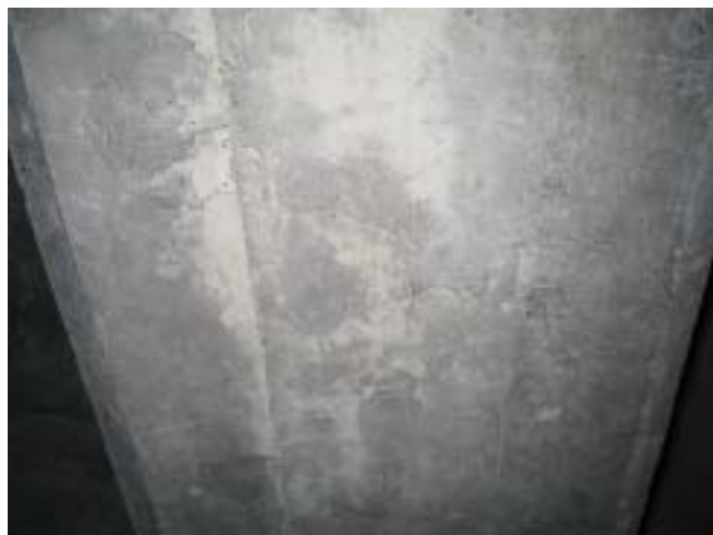
Fig. 4 Crack of main girder (Bridge A)
