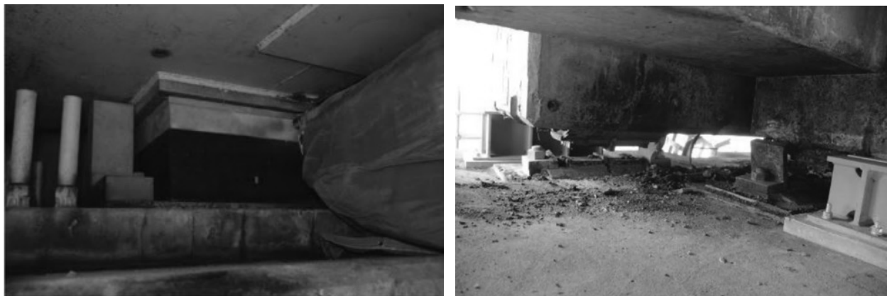
Fig. 2 (a) Undamaged Elastomeric Bearings and (b) Damaged Steel Pin Bearings
